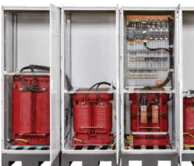
■ Test System for invertors
